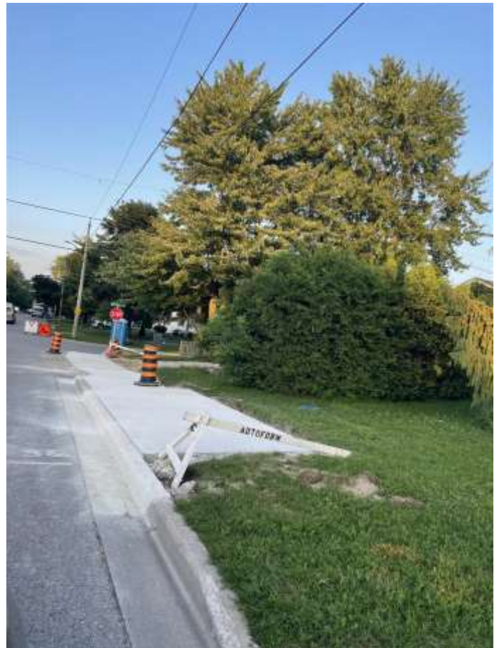
Picture 2 Corner of Eden Ave. and Easy St. - bus stop removed
